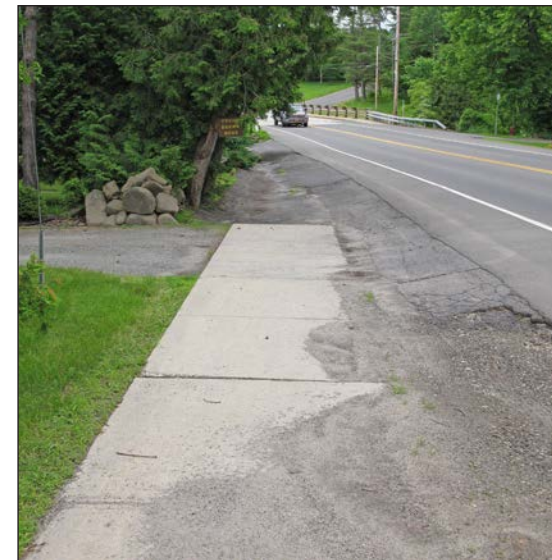
Evidence of stormwater problems at southern end of sidewalk
