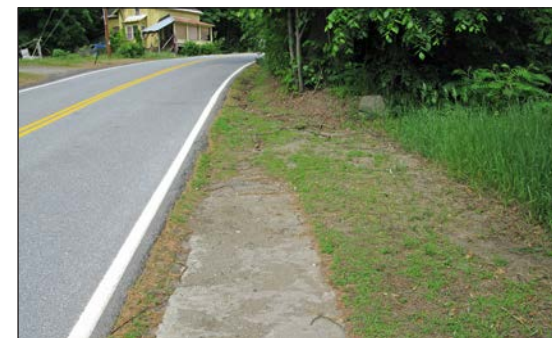
Sidewalk ends at blind curve
