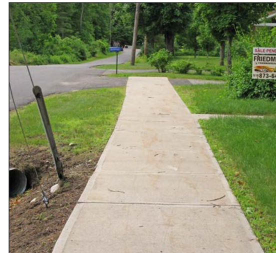
Looking at where the sidewalk ends on Foot Bridge Ln
