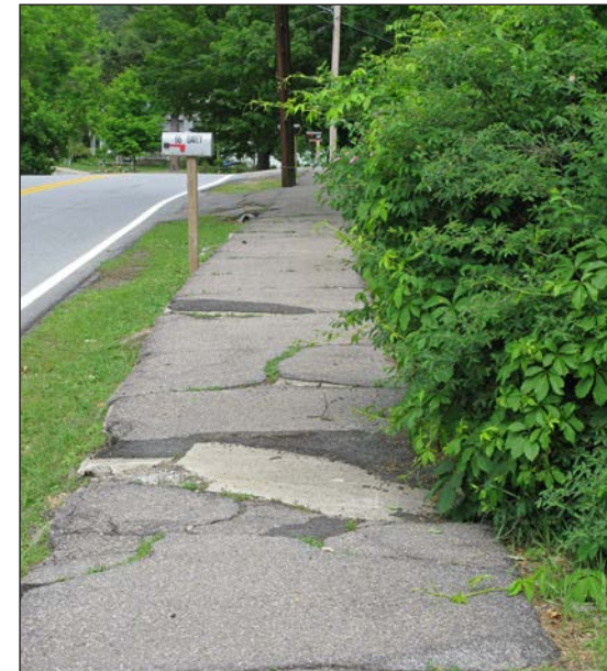
Deterioration and cracking of sidewalk
